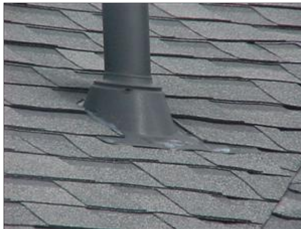
6.0 Picture 1 Main waste vent
